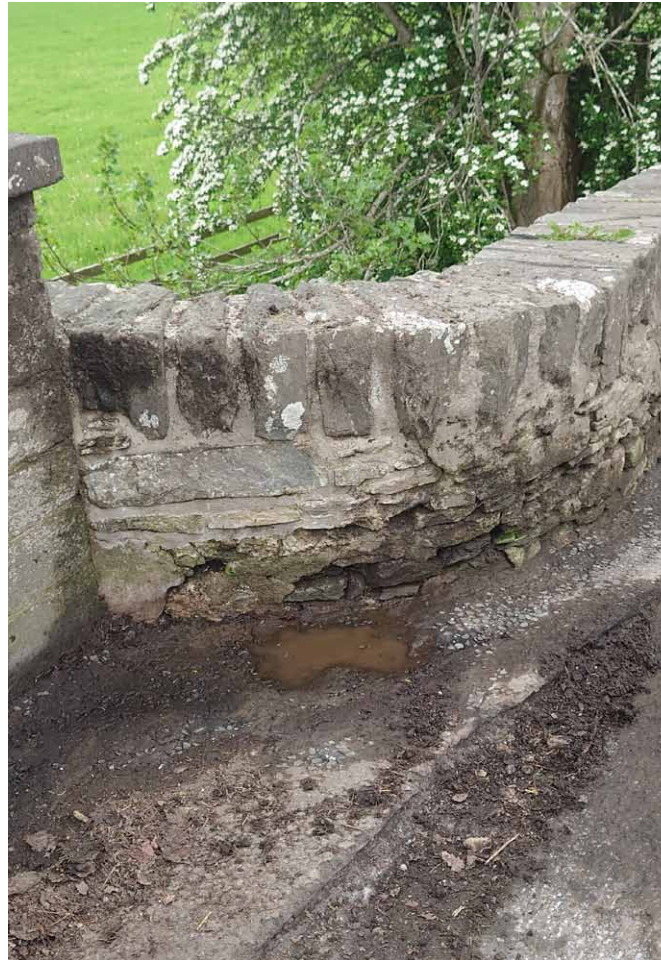
Inside face of upstream parapet wall showing eroded masonry and failed mortar pointing.
