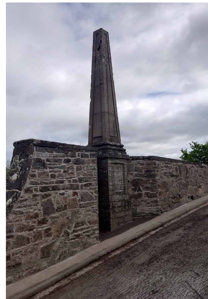
Inside face of downstream parapet wall showing eroded masonry, failed mortar pointing and inappropriate use of cement based mortar causing further deterioration to walls.
